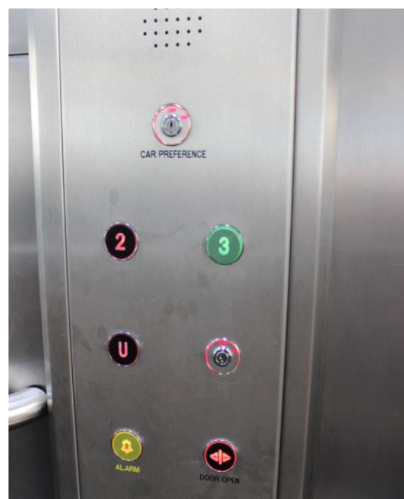
Lift buttons on lift on the Café side of the building.
