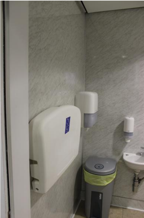
Photo of the baby change unit in the Accessible Toilets on the West side.
