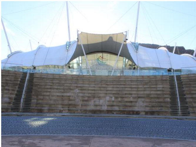
Step access from the amphitheatre to the main entrance, and the top of the stairs displaying the handrail and balustrade.
